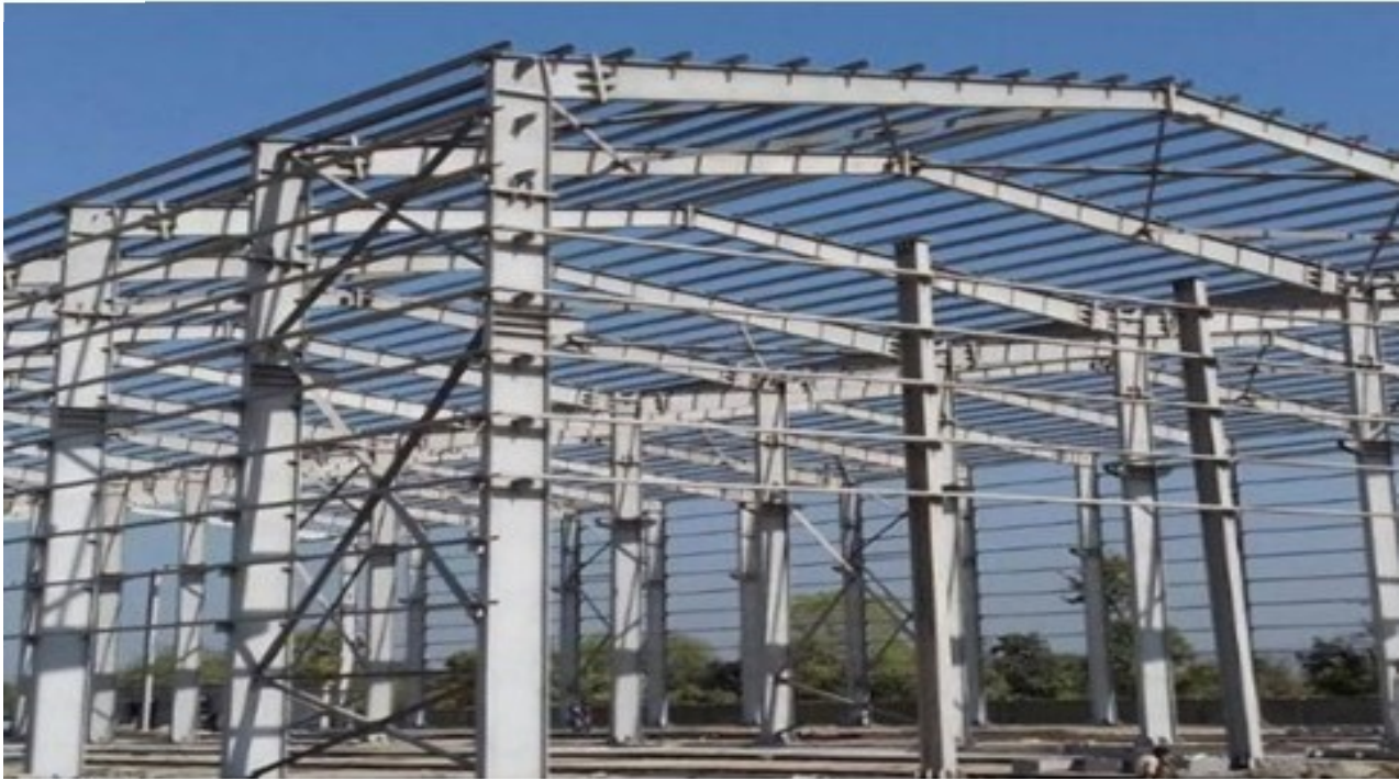
BODY & BOGIE REPAIR SECTION SHED AT SHAMBHUPURA, CHITTORGARH CLIENT : M/S OM PRAKASH GOYAL & CO.
